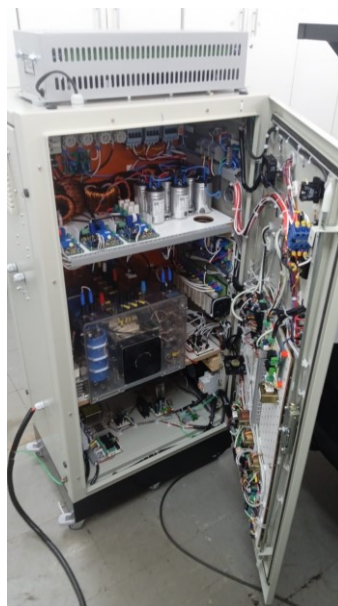
Figure 6.2 – Inverter unit inside.
