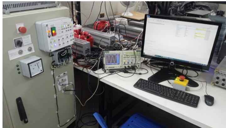
Figure 6.1 – Inverter unit operating.
