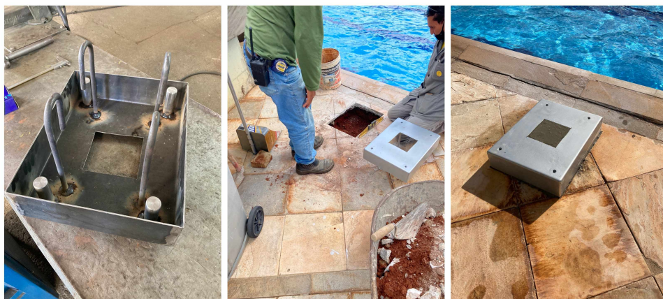
Figure 19 – Anchoring base and concrete slab being mounted in the edge of the pool.
