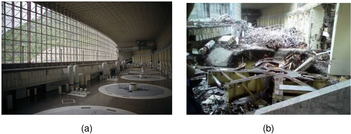
Figure 1.1: Turbine hall of the power station: (a) before, and (b) after the accident. Source: http://4044415.livejournal.com/51884.html
